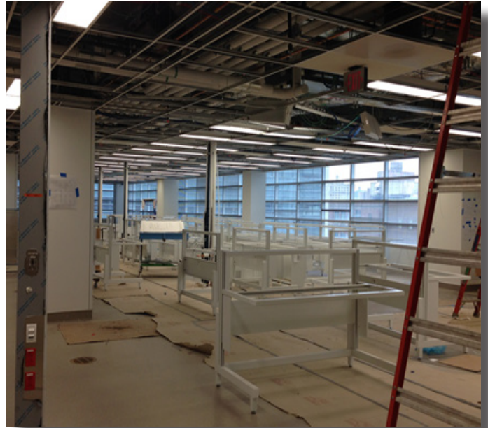
A northeast view of the new Core Laboratory, 4th floor, IOH Building.
